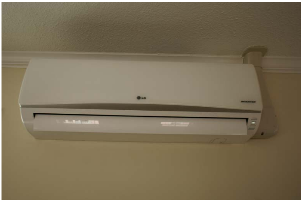
LG Remote Control HVAC System
